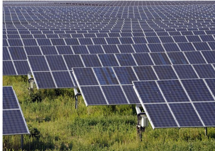
Example of rows of solar panels.
